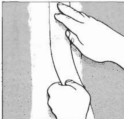
6 Once the entire joint is covered smoothly with compound, cut a piece of tape and embed it in the compound over the joint line.
