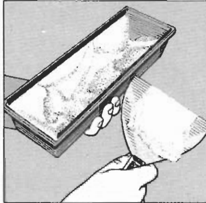
4 Begin work on the butt joints by loading a 5-in. knife with compound. Scrape the excess compound off both corners of the knife.
