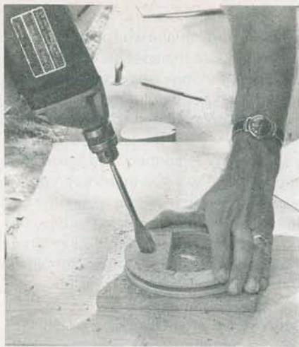
Fig. 6. Drill shaft hole with wood bit, tilting it away from D cutout by about 18 degrees.
