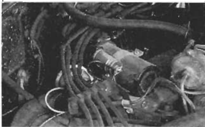
Fig. 3 (top) Drawing of ignition coil terminals, cables, and proper placement of coaxial capacitor. (Bottom) Spark coil with coaxial capacitor securely attached and grounded to coil's mounting strap.
