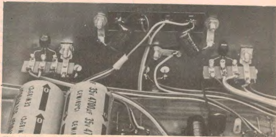
This photograph shows how the thermal compensation transistors are mounted.
